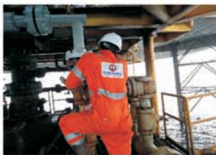
INSTALLATION OF FLOW LINE IN PROGRESS BY EVERPRAISE ENGINEER AT UKPOKITI OFFSHORE
