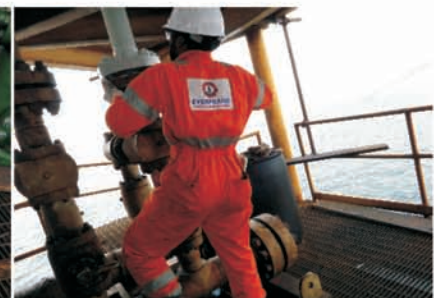
INSTALLATION OF NEW FLOW LINE ON THE EXISTING MANIFOLD BY EVERPRAISE ENGINEER AT UKPOKITI OFFSHORE
