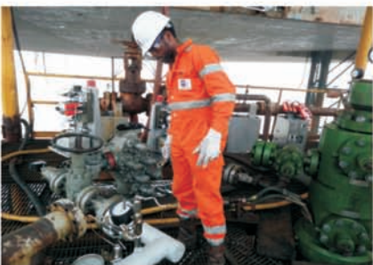
FLOW LINE SPOOL PIECE TIED TO XMAS TREE GATE VALVE
