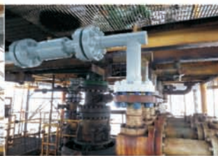
NEW FLOW LINE INSTALLED BY EVERPRAISE ENGINEER AT UKPOKITI OFFSHORE
