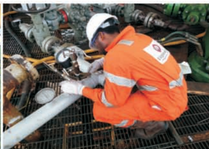
INSTALLATION OF FLOW METER AND THERMOWELL ON THE FABRICATION FLOW LINE BY EVERPRAISE
